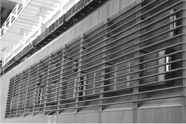
FIG.6 Side mounted coolers
